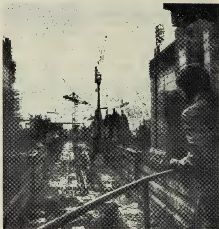
Work on the large Iron Gate hydropower site is at an advanced stage. In the picture: "The main line" in the waterlock
